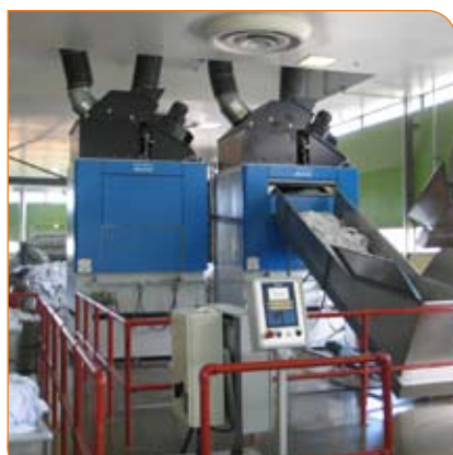
The two Jensen dryers installed at CLS.
